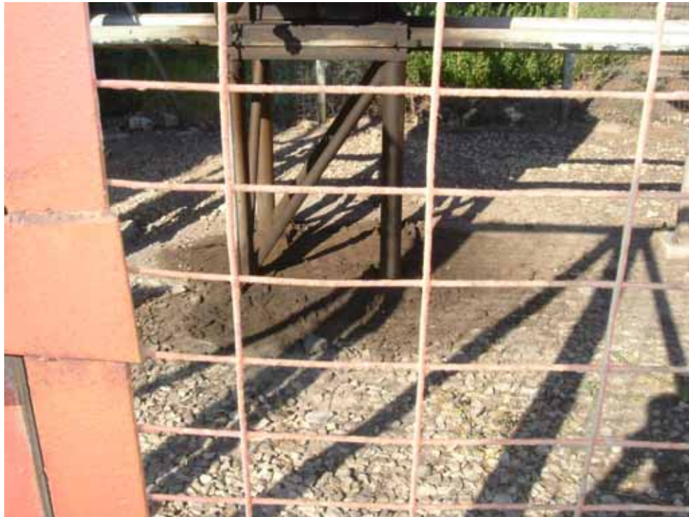
Hydrocarbon Staining Under Transformer Near to TP38
